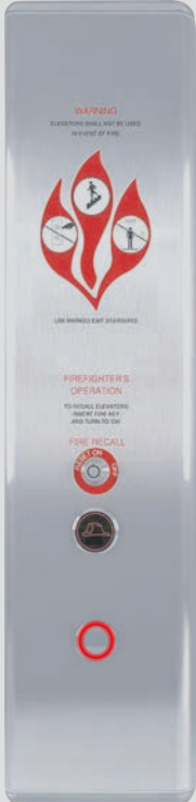
Hall pushbutton with fire recall
