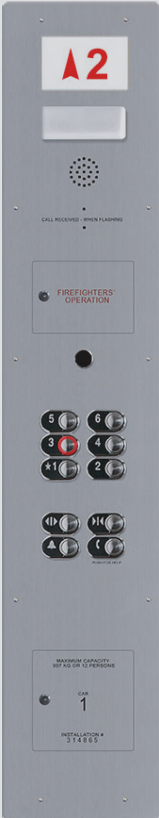
Car operating panel
